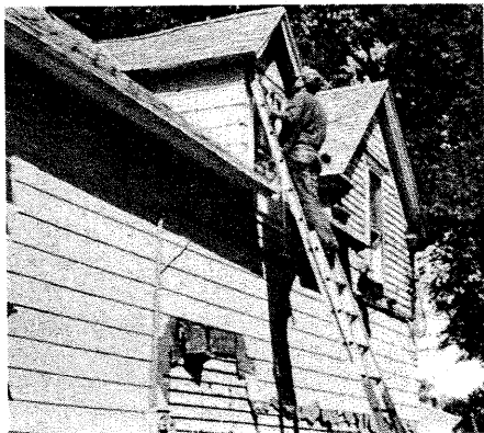
Current rehabilitation of 693 Conway Street includes restoration of the original wood siding. From 1914 to 1933 this was the home of Warren Burger, the former Chief Justice of the U.S. Supreme Court. The simple gable roofed house was built in 1884 for $2,000.
