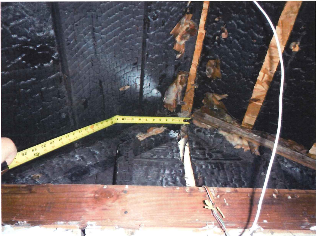
Photo 2- Gap between rafters and wall sheathing on west end of roof
