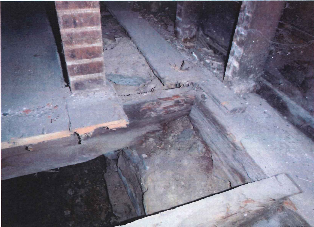
Photo 7- Deteriorated joists and sill at bearing on stone foundation wall
