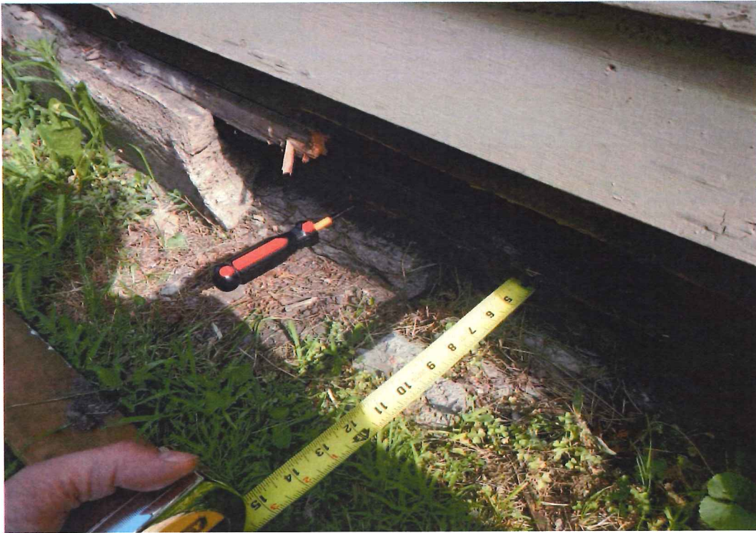
Photo 5- Rotted wood and missing/deteriorated stone materials at base of stud wall
