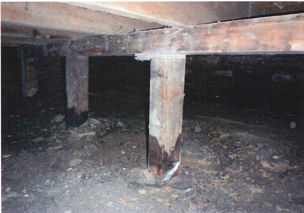
Photo 8- Signs of moisture on columns in crawl space
