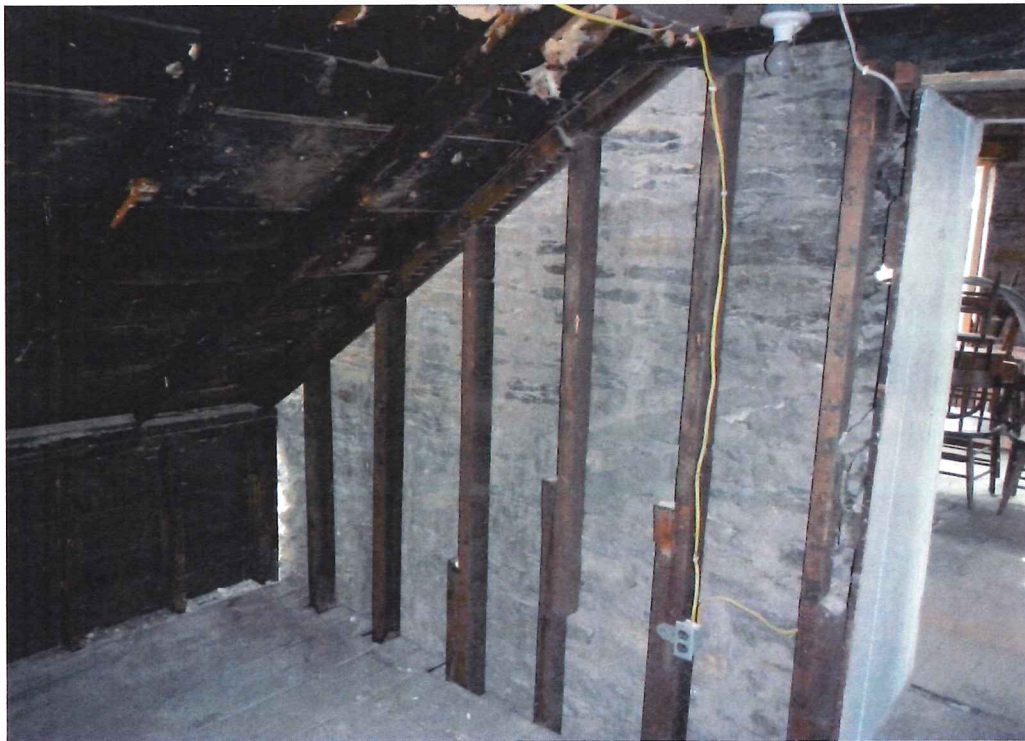
Photo 10- Sistered wall studs along east gable end at previous remodeling efforts
