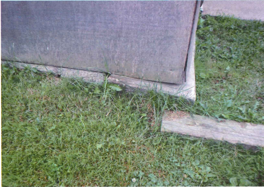
Photo 9- Signs of movement in concrete supporting stud walls of one story shed on west side of building
