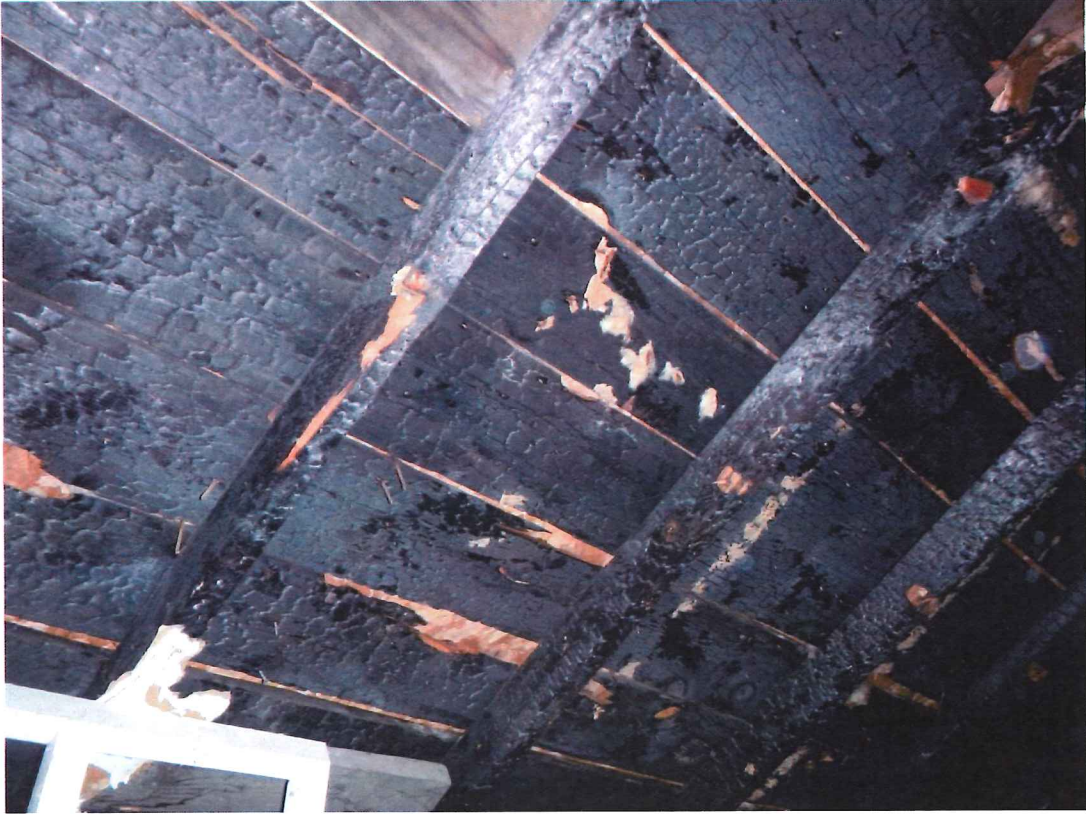
Photo 1- Fire damage at roof level
