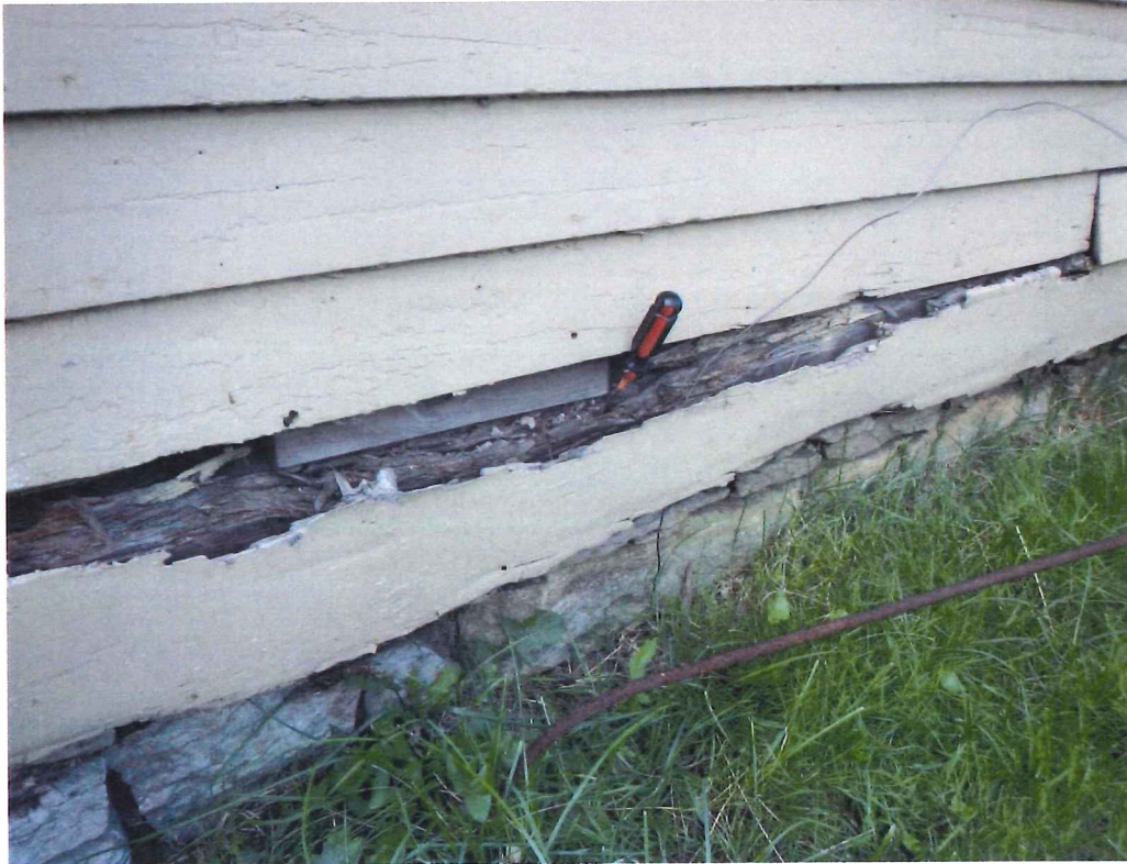
Photo 4- Rotted wood and deteriorated stone materials at base of stud wall
