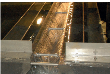
Filters during backwash.
