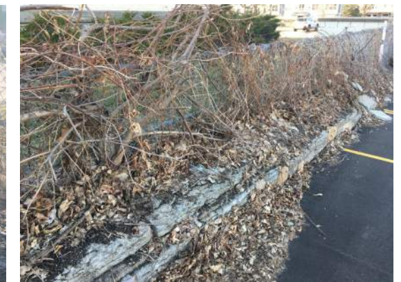
Existing Wall @ East Elevation (Erroded)
