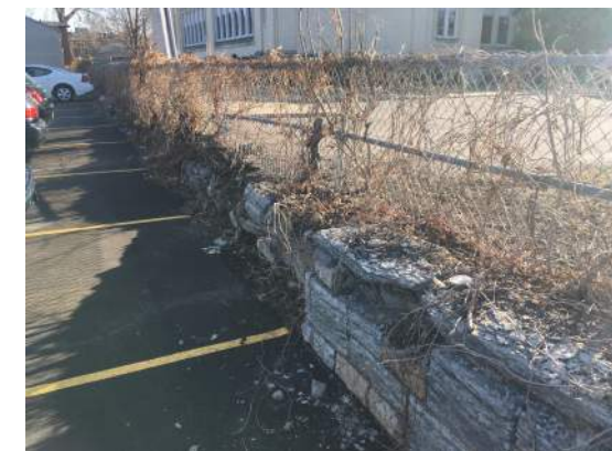
Existing Wall @ East Elevation (Erroded)
