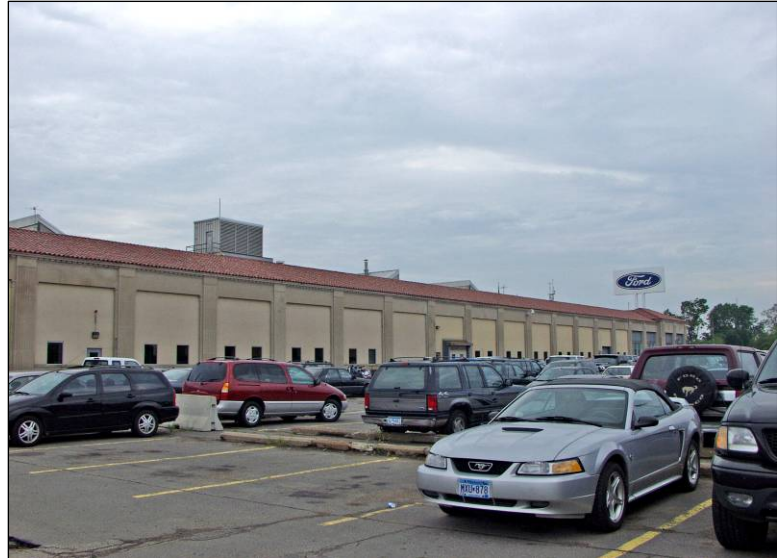
Window openings on the north facade of the main assembly building have been enclosed with concrete block.
