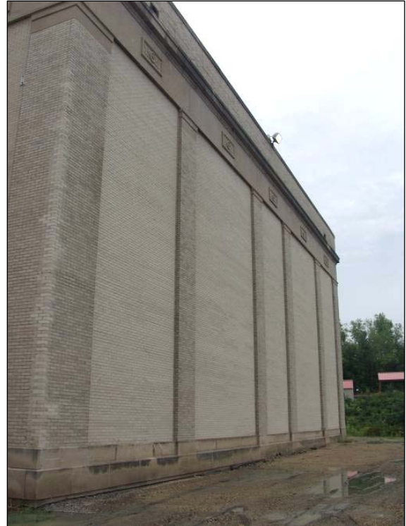
The window openings on the west facade of the steam plant were enclosed following flooding in the 1950s.
