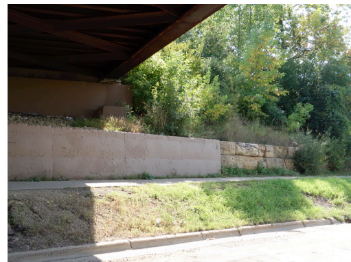
Figure 5. Stone and concrete retaining wall, under CM& StP Railway Bridge No. 92258, at Prior Avenue N.
