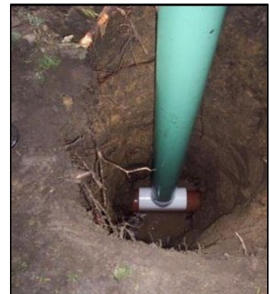
Exterior cleanout pipe (green) attached to sewer lateral in newly dug hole.
