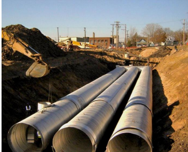
Photo 4-1: Underground Infiltration Chamber (Facing West)
