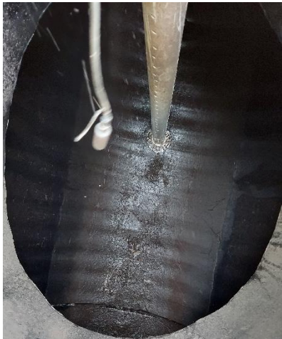
Photo 2-1: Infiltration Gallery Level Monitoring Enclosure
