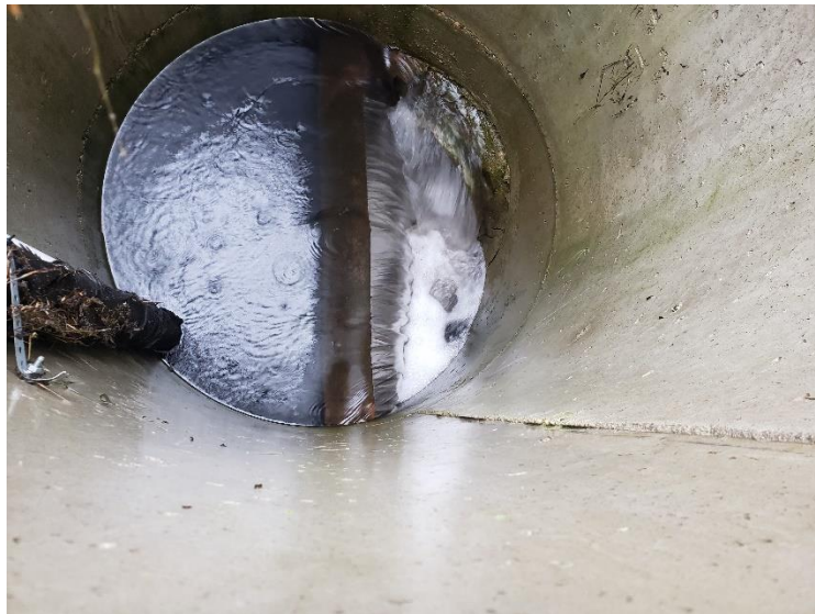
Photo 4-3: Water being conveyed back to the storm sewer from the underground chamber in the outlet control structure.
