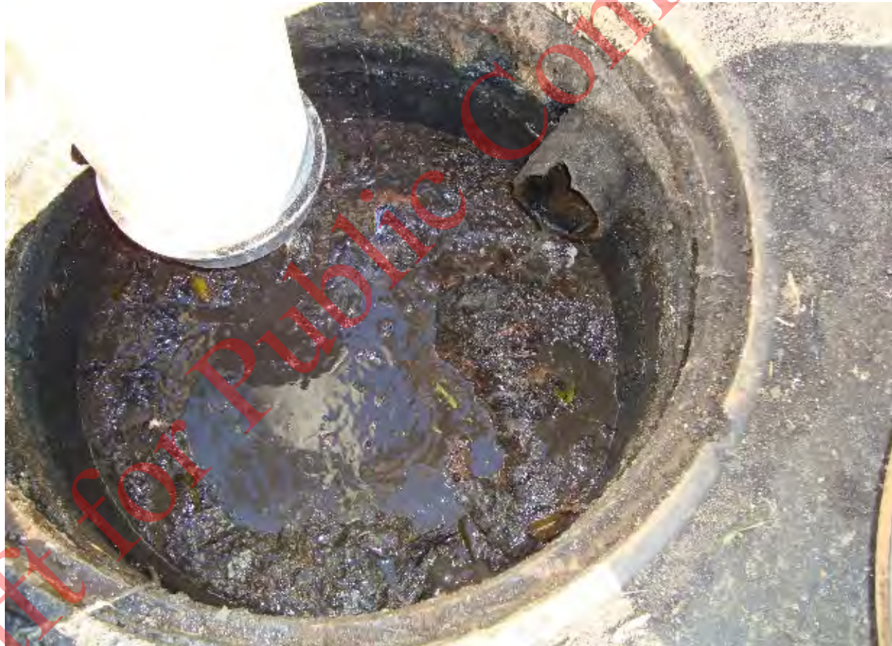
Sanitary Discharge, Private Storm Drain
