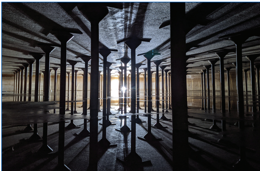
Hillcrest reservoir after crews cleaned out the facility in 2021. Reservoirs get cleaned out with maintenance work completed as needed.
