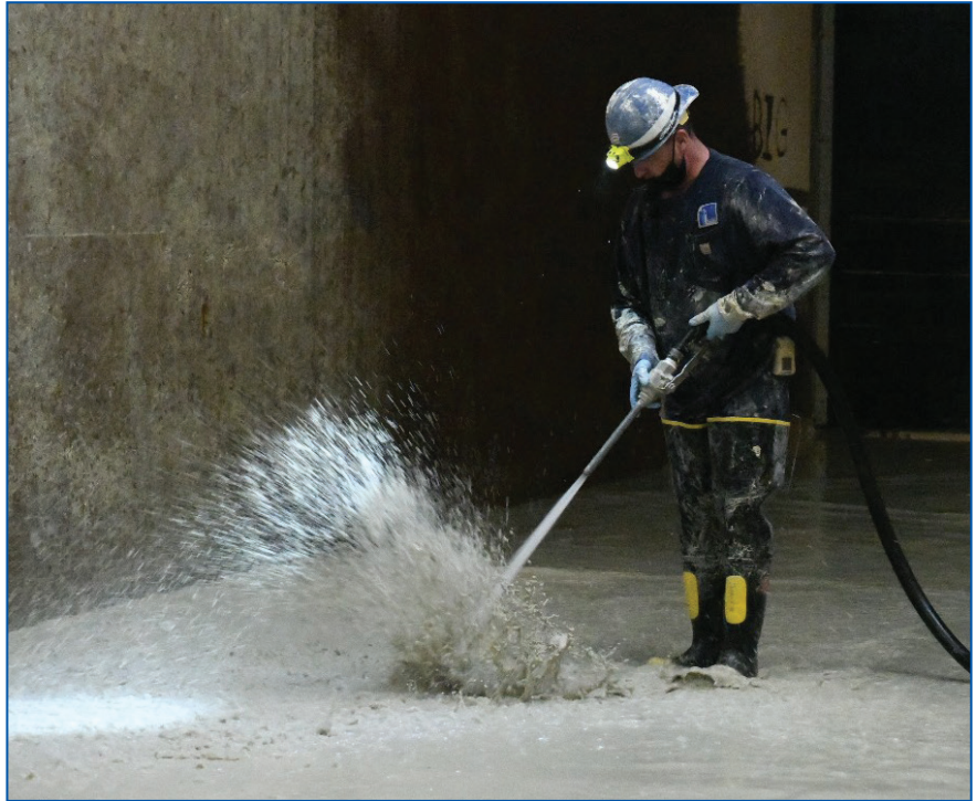
A worker cleans out the re-carb basin in the McCarrons treatment plant.
