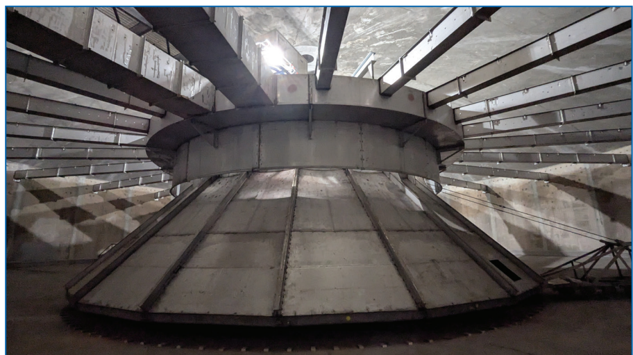
The interior of one of the clarifiers in the new water treatment plant.
