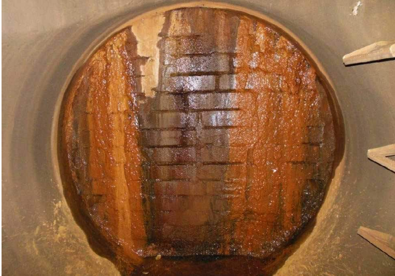
Iron Bacteria on Bulkhead
