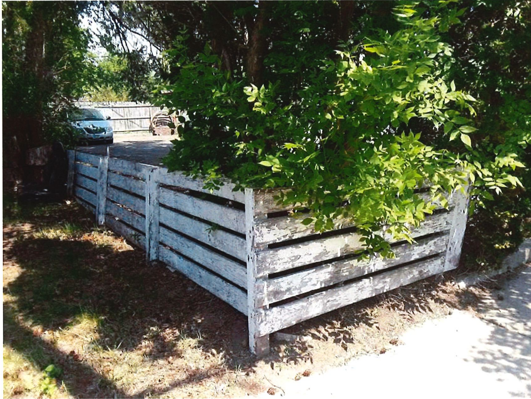
Subject property – condition of fence
