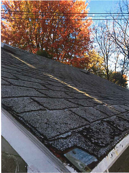
Roof, both the ridge and rafters sag
