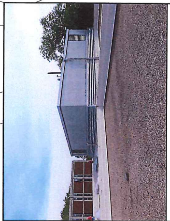
SOUTH EQUIPMENT LOCATION [LOOKING NORTH]
