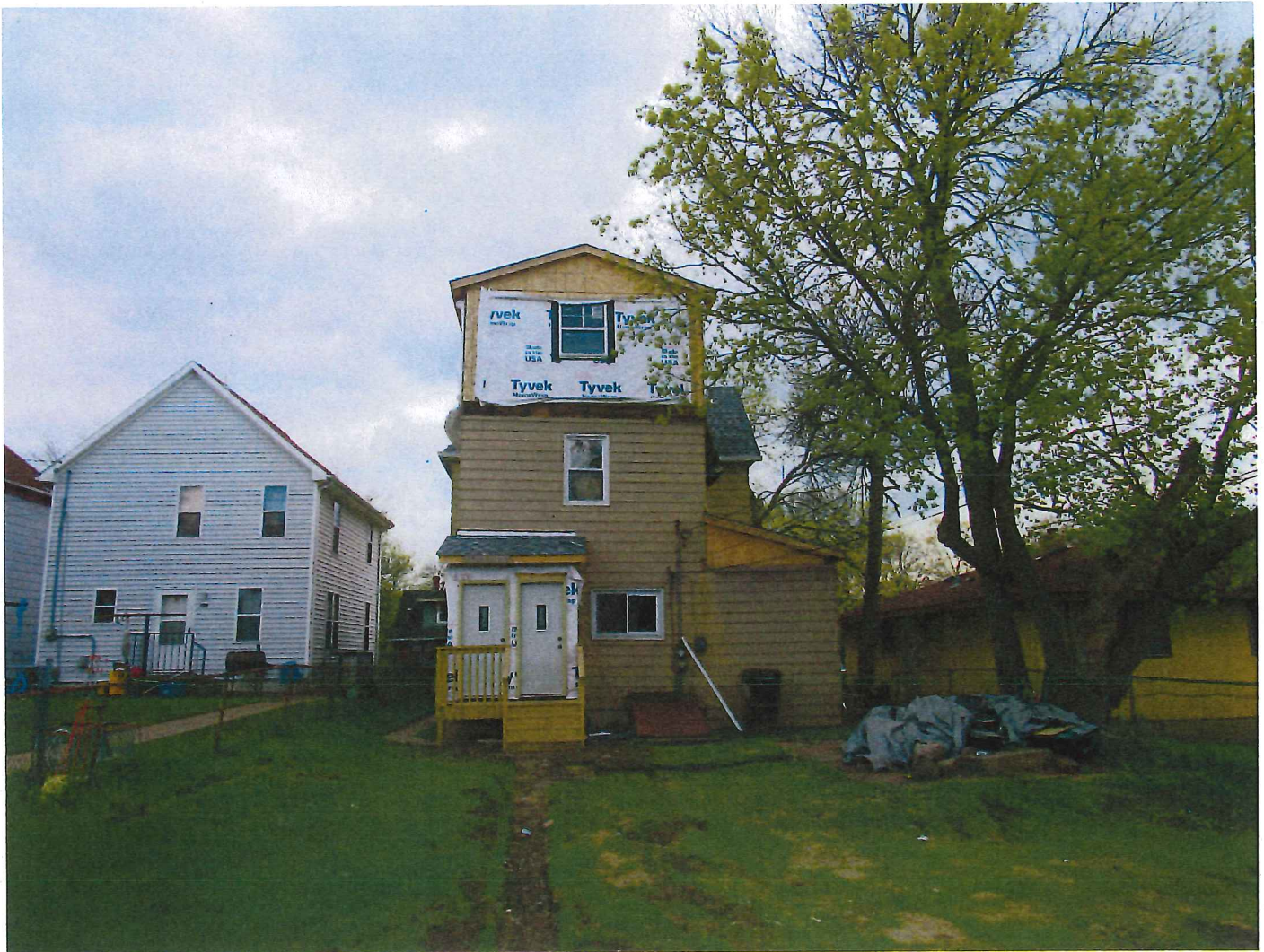
Rear third floor addition constructed without permit approval from the Department of Safety and Inspections.
