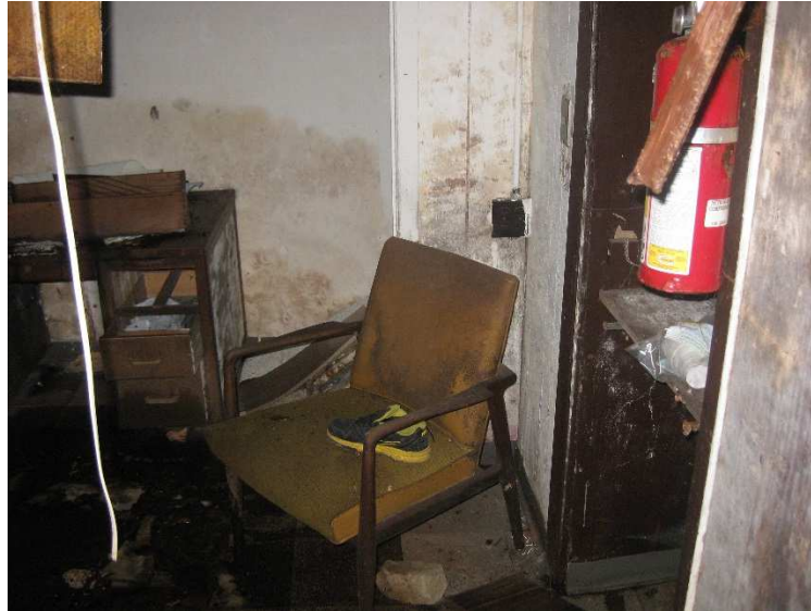
Picture 2 – Water Damage to Walls
