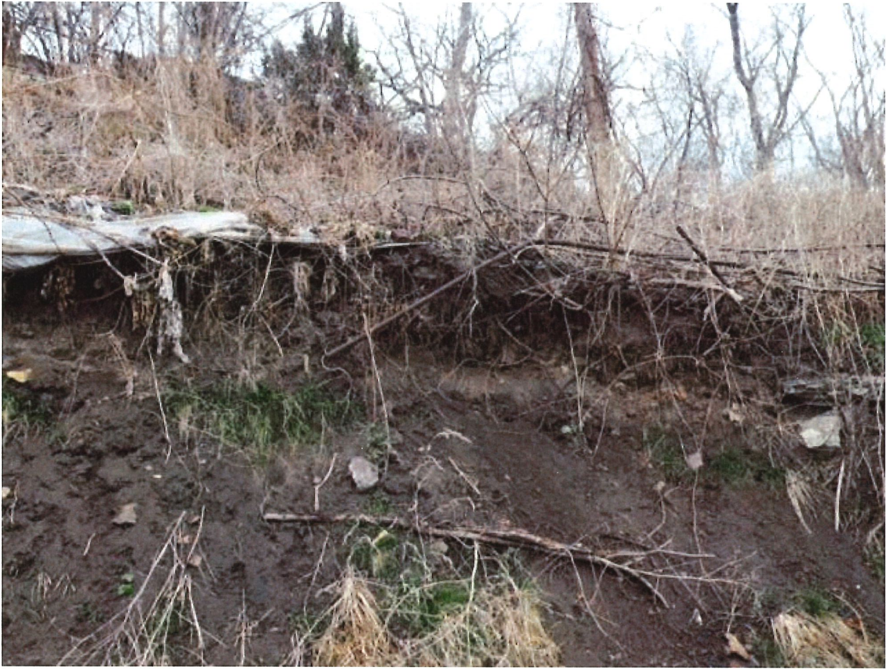
Unstabilized soil below 322/324 Summit
