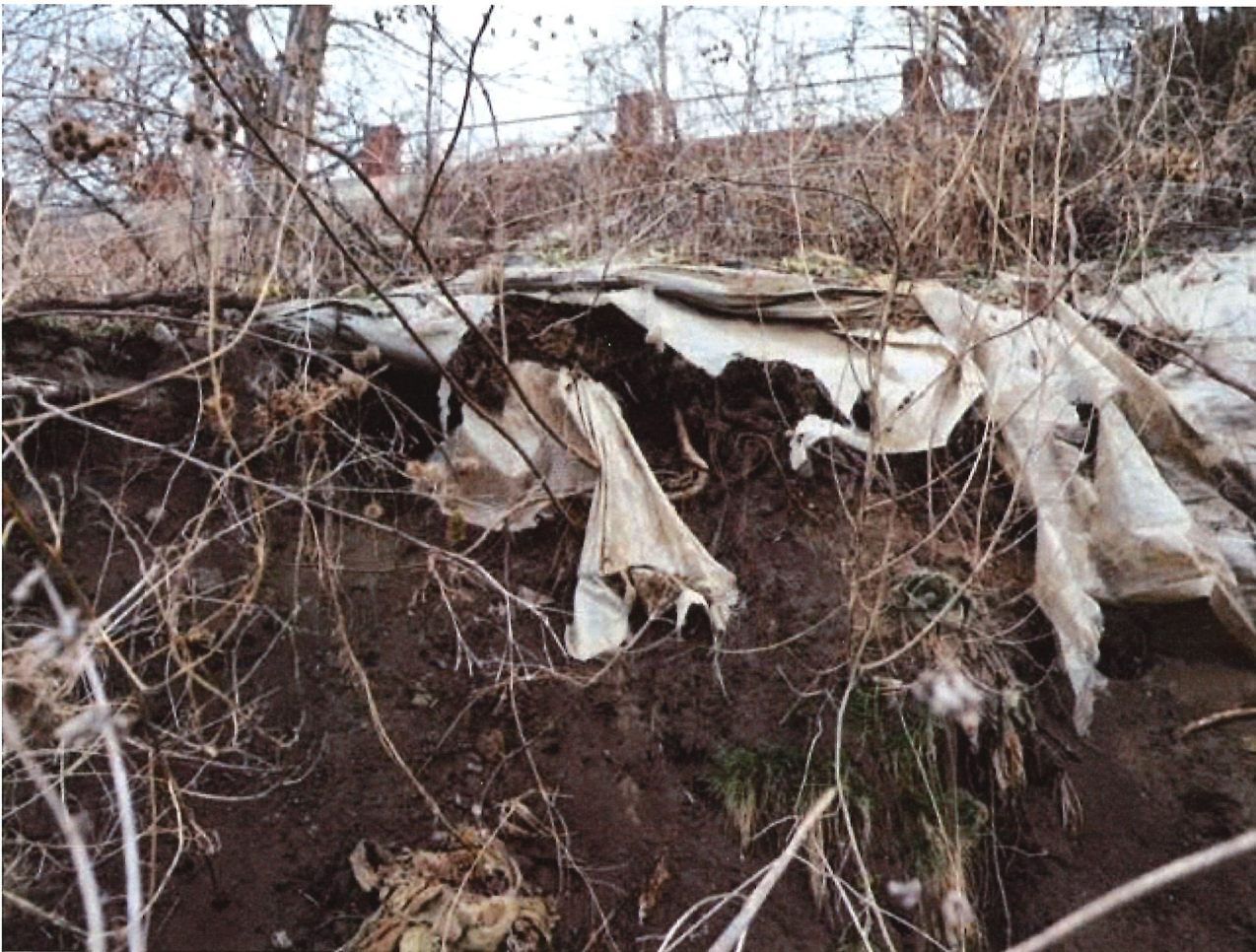
Backhoe destruction of soil retention fabric
