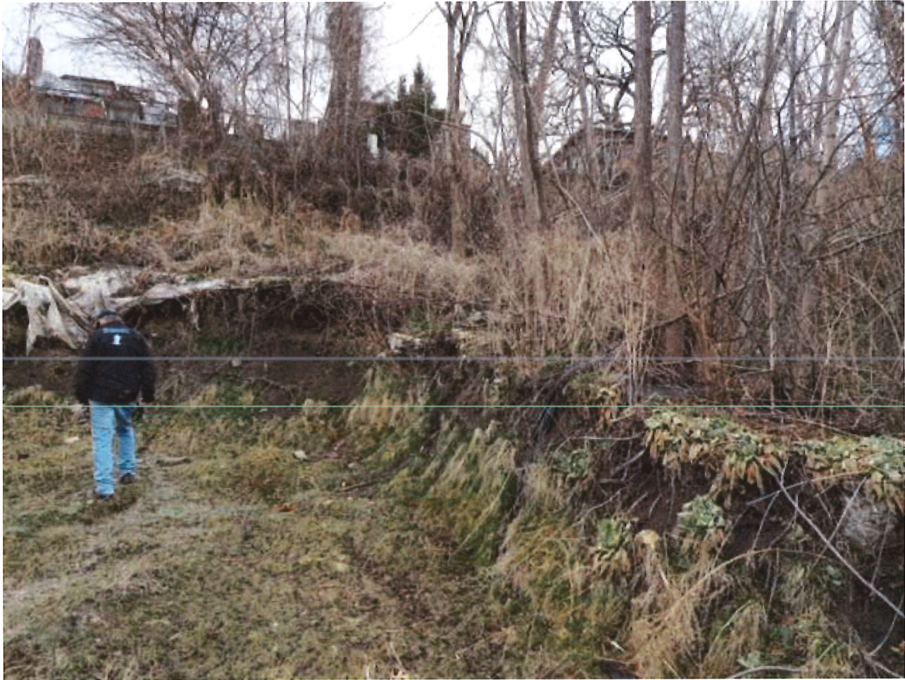
Vertical cut in slope below 322/324 Summit
