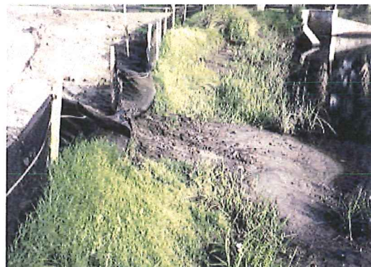
Silt fence that was not maintained
