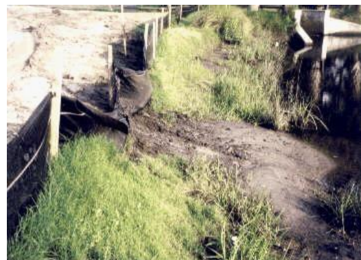
Silt fence that was not maintained
