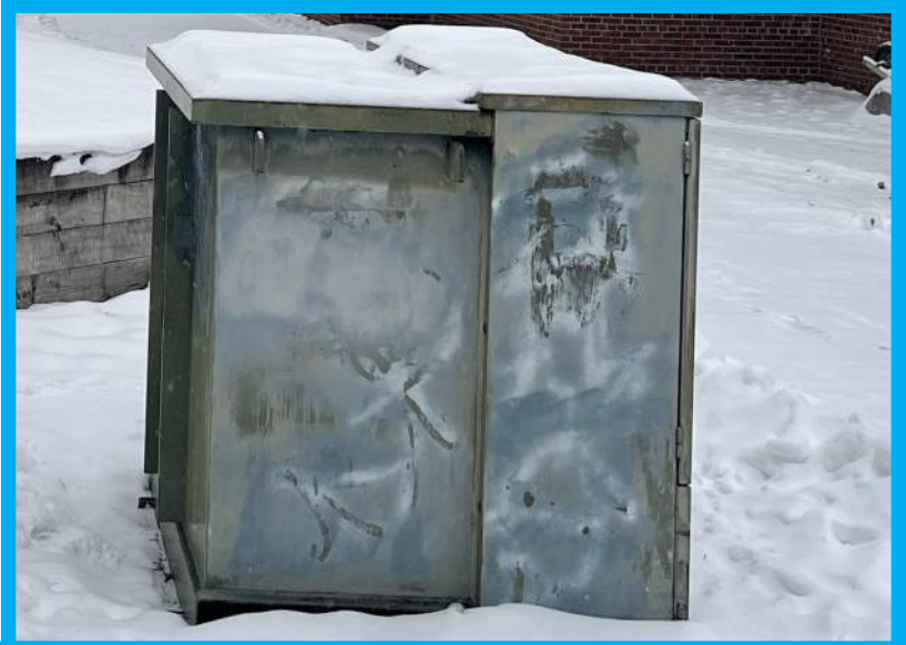
Art Location 1 - Electrical Transformer
