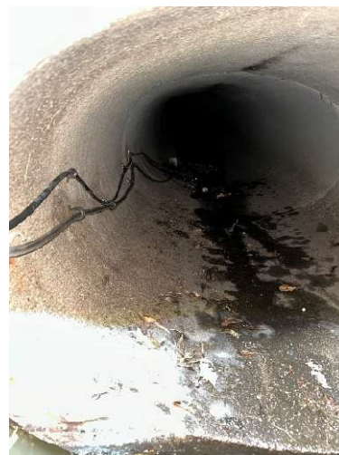
Photo 2-2: Sensor configuration in St. Albans elliptical pipe
