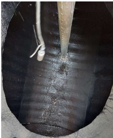
Photo 2-1: Infiltration Gallery Level Monitoring Enclosure
