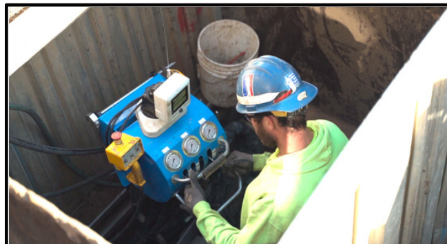
A worker guides horizontal drilling equipment underground to allow for a new copper line to be pulled through from the street to the house during a lead replacement.
